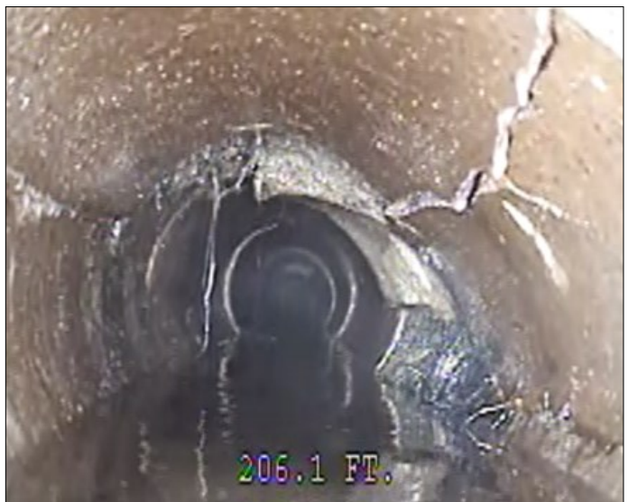
Many pipes in the Rocky Ford wastewater system are subject to infiltration and in need of replacement.
